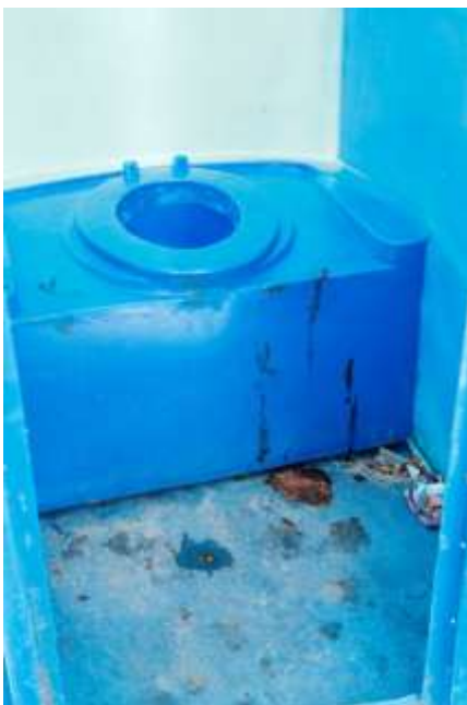
Uncleaned chemical toilets Photo: Sowmya Kidambi
